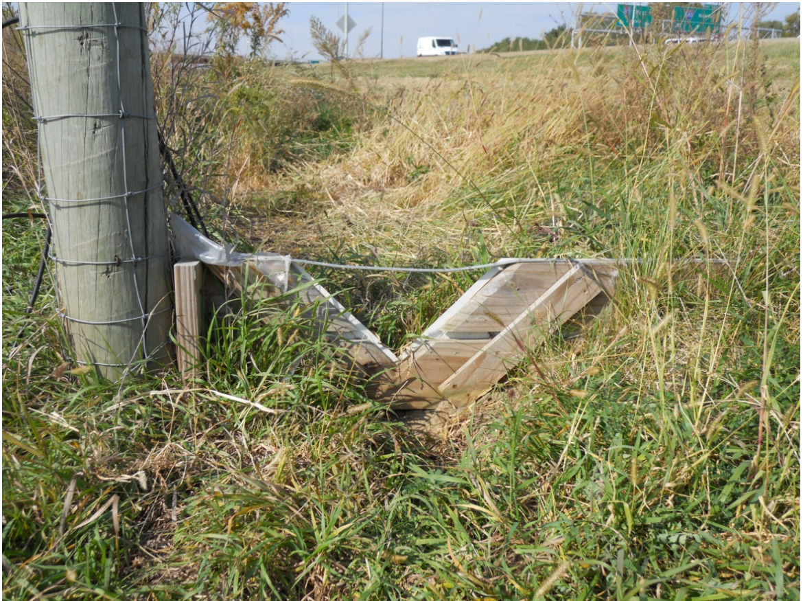
Figure 4-4: V-Notch Weir Installed at Site B
