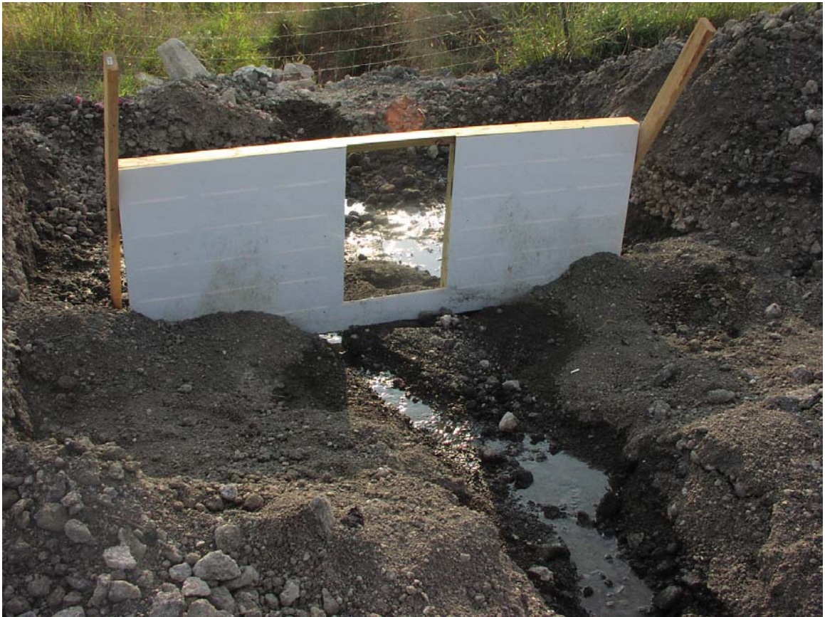
Figure 4-3: Rectangular Weir Installed at Site A
