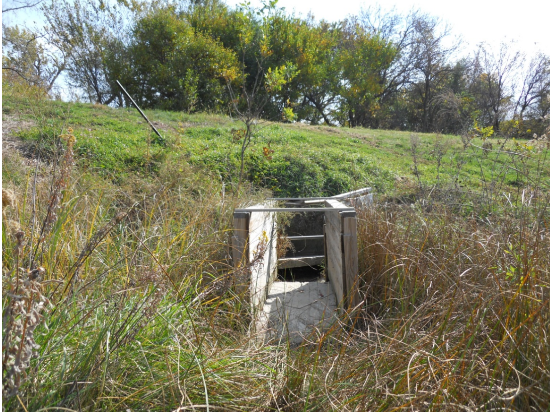
Figure 4-5: Rectangular Flume Installed at Site E
